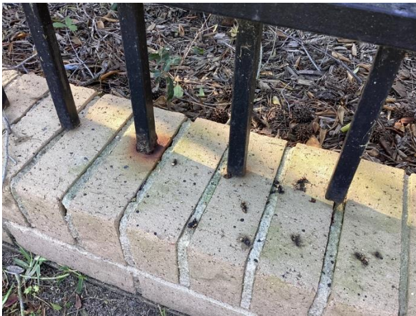
Fence finish deterioration
