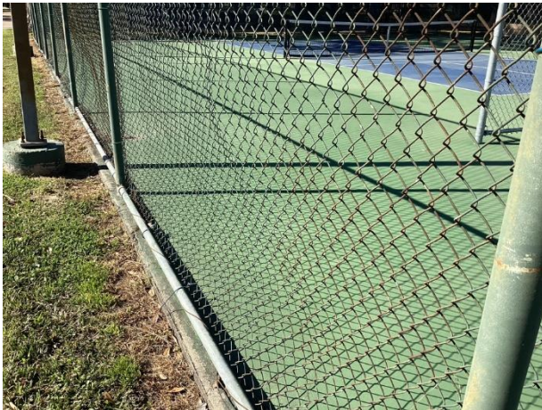
Chain link fence with warped webbing
