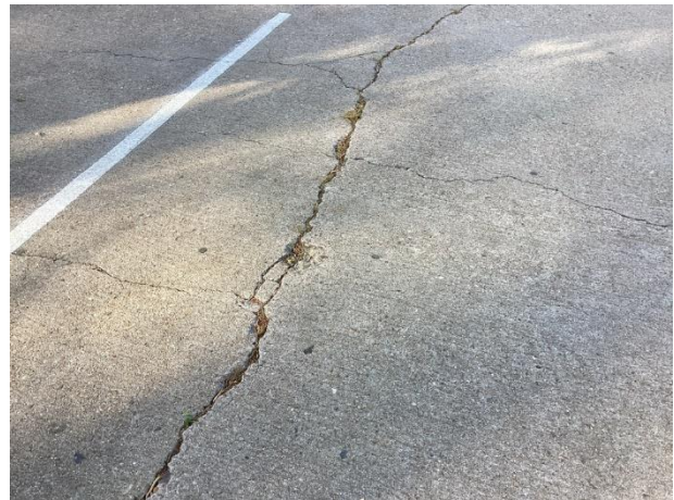
Cracks and spalls
