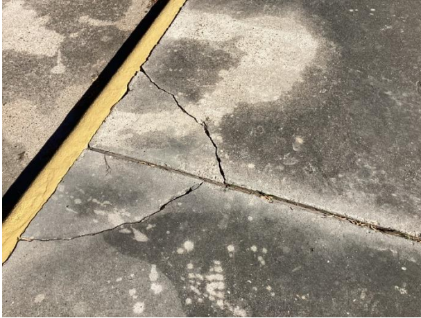
Concrete sidewalk with cracks
