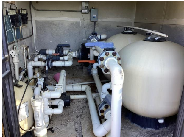
Pool mechanical equipment Pinehurst
