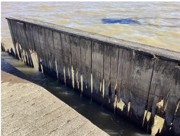
Wood bulkhead with wood rot and deterioration
