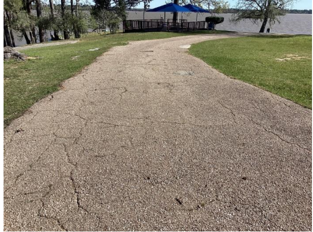
Pavement overview with cracks
