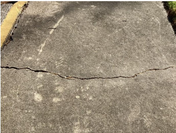
Concrete sidewalk with crack
