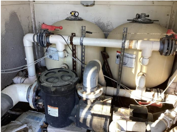
Pool mechanical equipment shores
