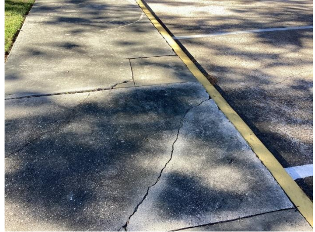
Concrete sidewalk with cracks
