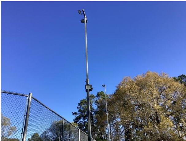
Light pole and fixture
