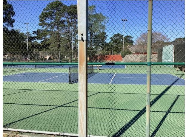
Pole finish deterioration
