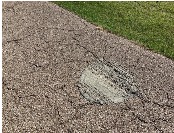
Pavement overview with cracks
