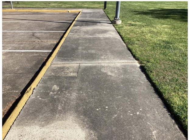
Concrete sidewalk with partial replacement
