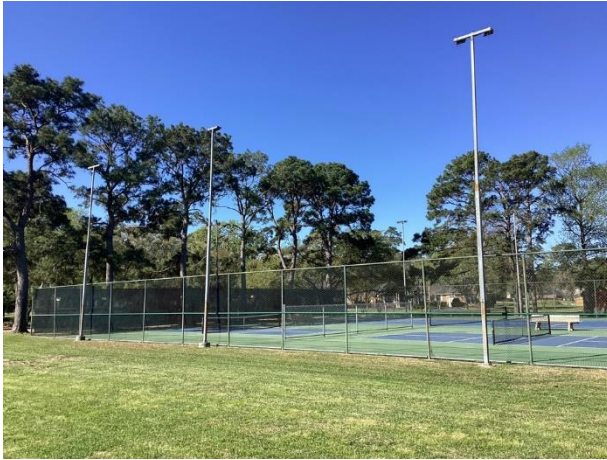
Light poles and fixtures
