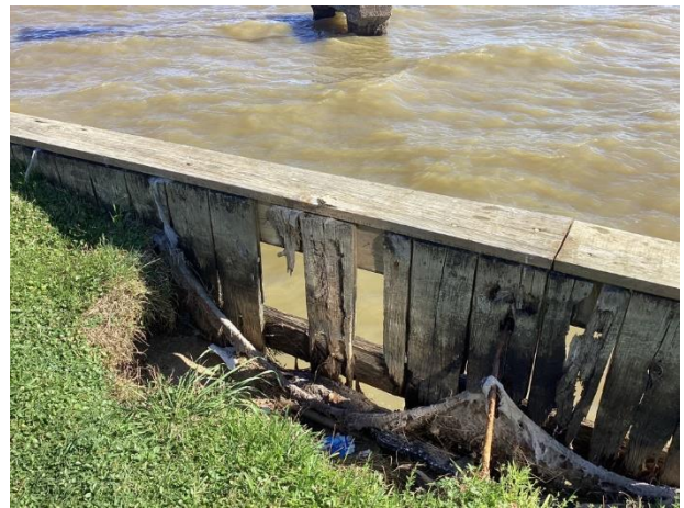
Wood bulkhead with wood rot and deterioration
