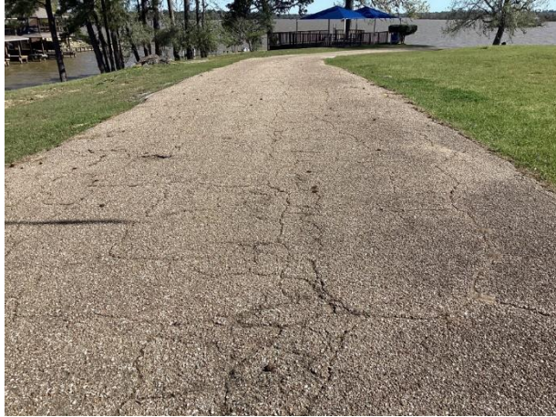
Pavement overview with cracks
