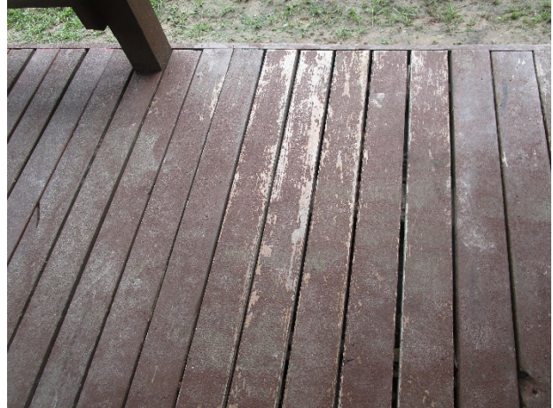
Deck board finish deterioration
