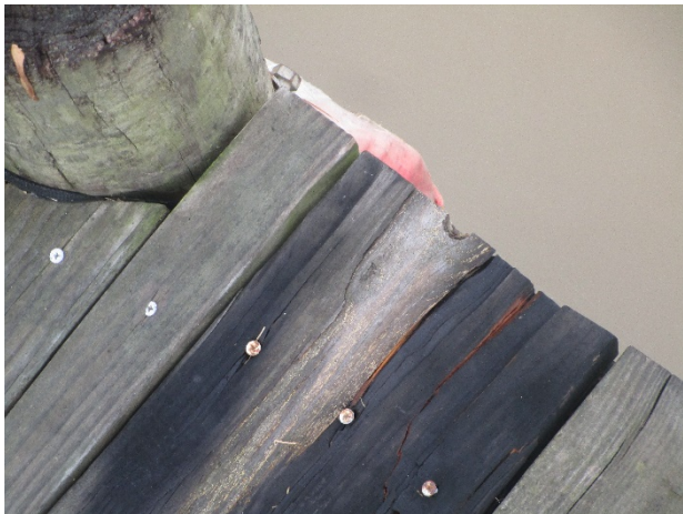
Deck board wood rot at the walkway
