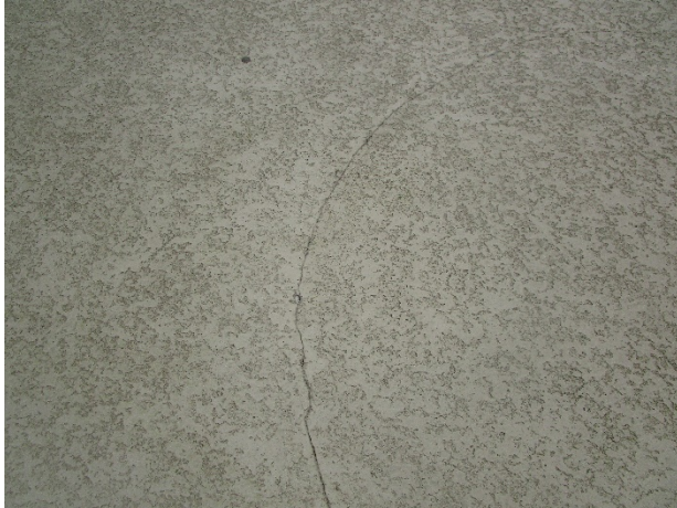
Cracks at the Shores pool deck
