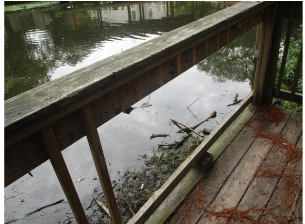
Missing and damaged rails
