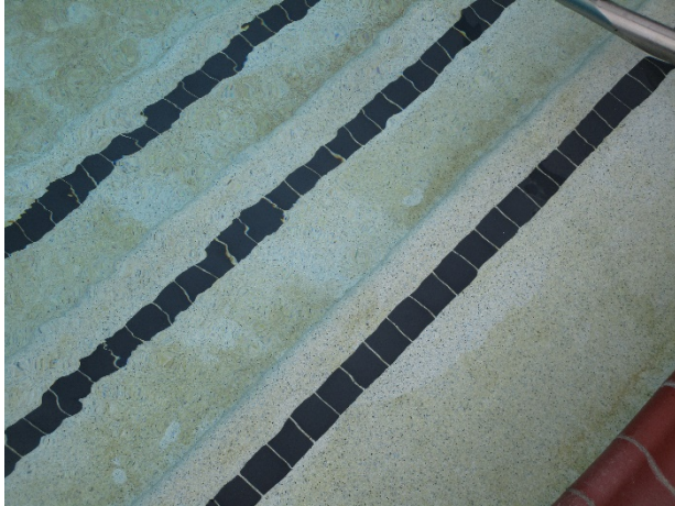
Plaster deterioration at the Pinehurst pool
