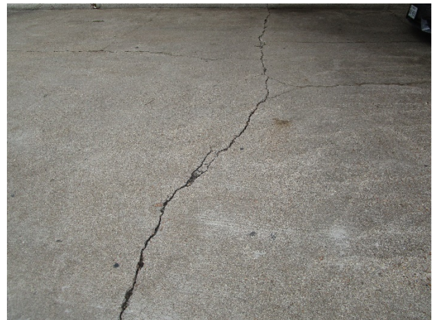
Parking area cracks at the Shores pool
