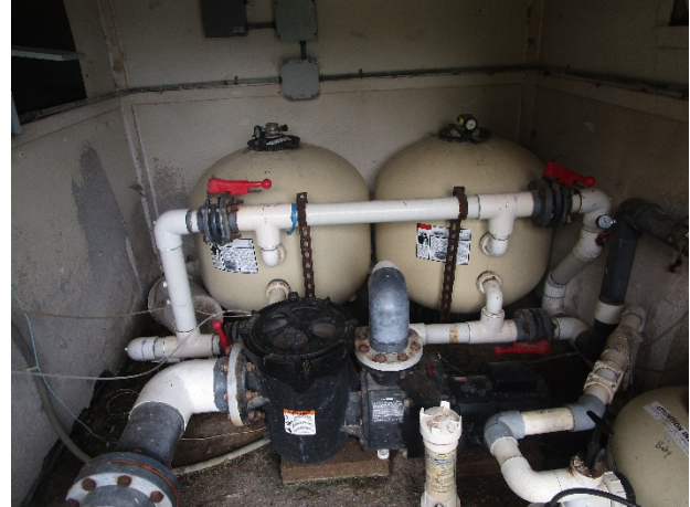
Shores mechanical equipment overview
