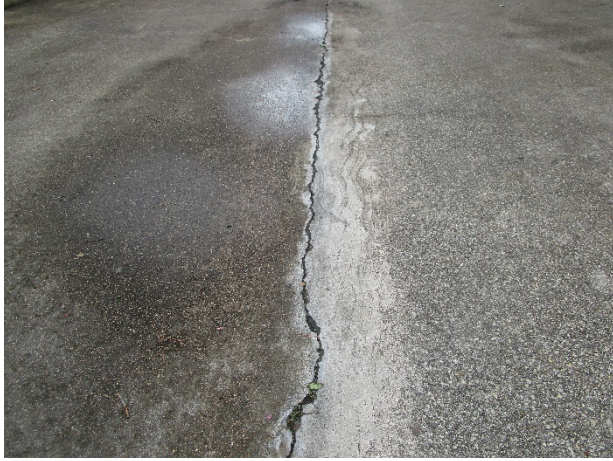
Parking area cracks at the Shores pool
