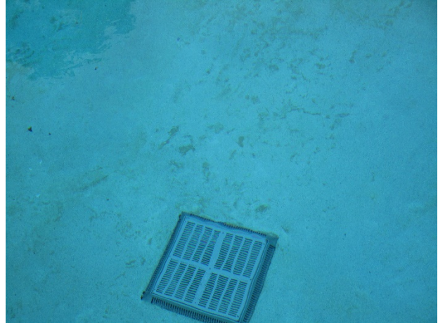
Plaster deterioration at the Pinehurst pool
