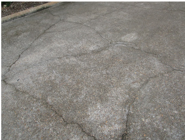
Parking area cracks at the Shores pool
