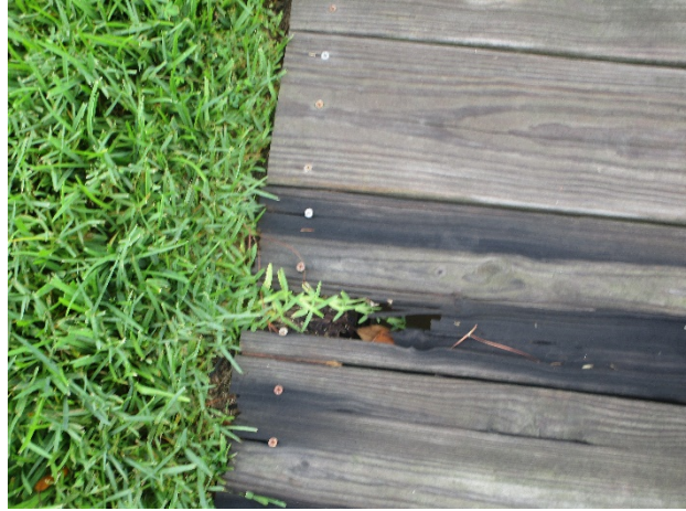
Deck board wood rot at the walkway
