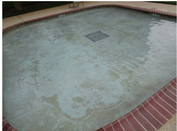
Plaster deterioration at the Shores pool
