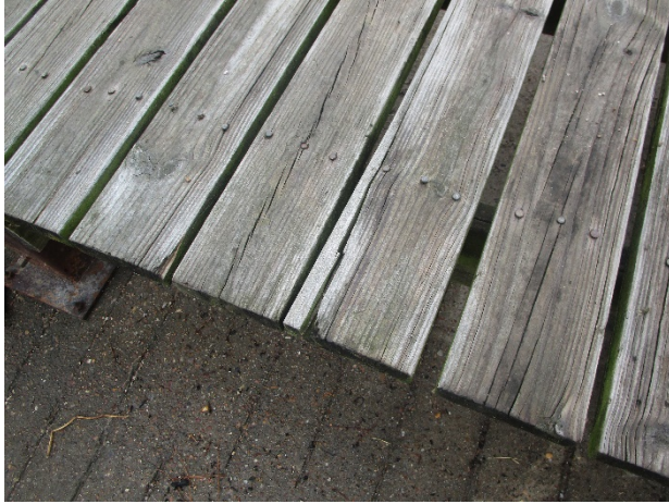
Split wood deck board at the dock
