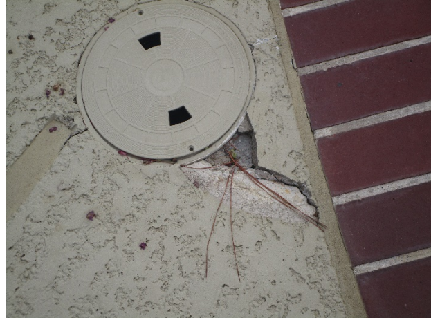
Cracks at the Shores pool deck
