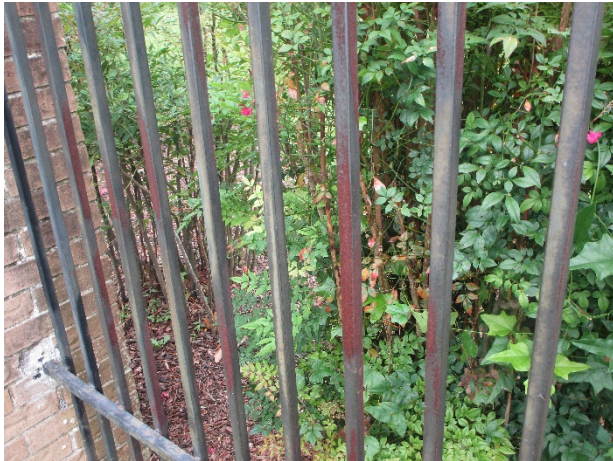
Rust at the Shores pool fence
