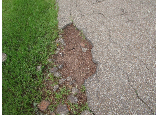
Pot hole and pavement deterioration
