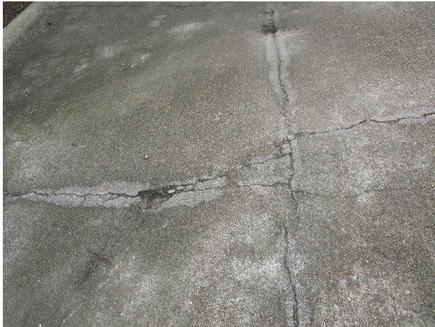
Parking area cracks at the Pinehurst pool
