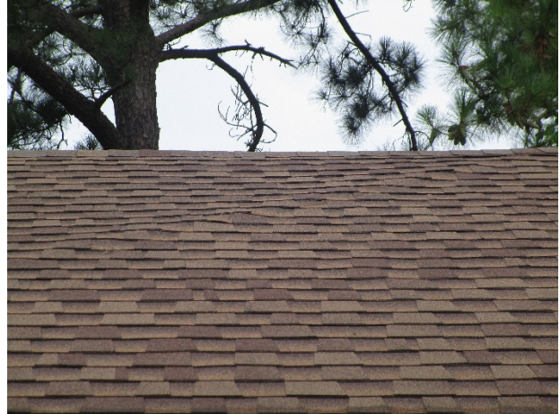
Sheathing deflection and minor shingle lift at the Pinehurst pool house roof
