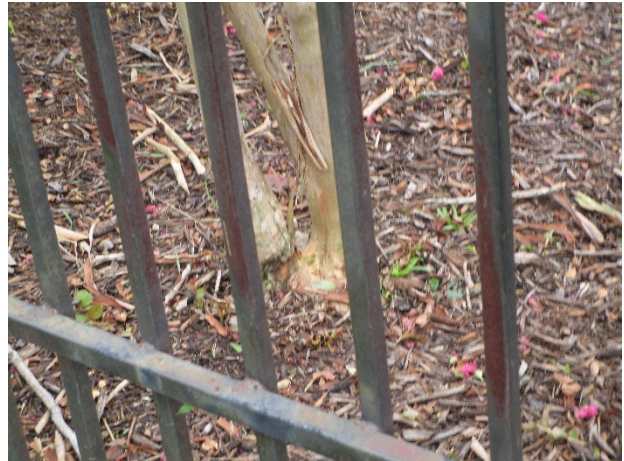
Rust at the Shores pool fence
