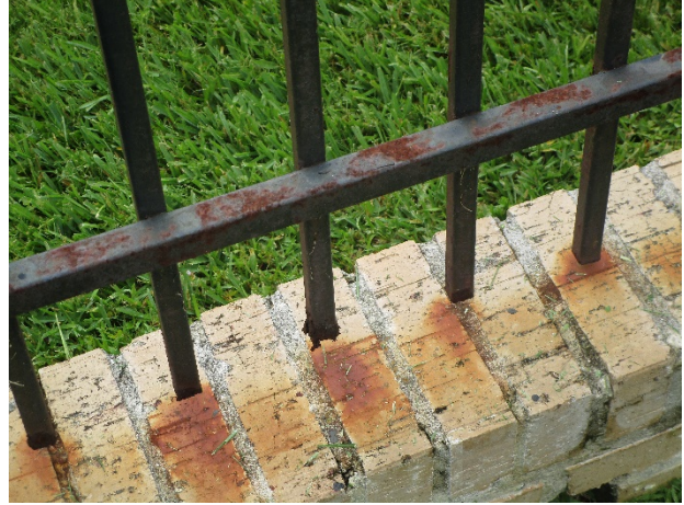
Rust at the Pinehurst pool fence
