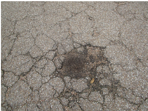
Pavement cracks and deterioration
