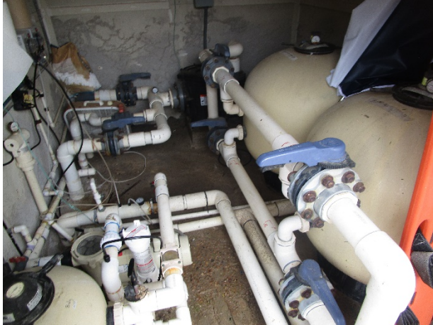
Pinehurst mechanical equipment overview
