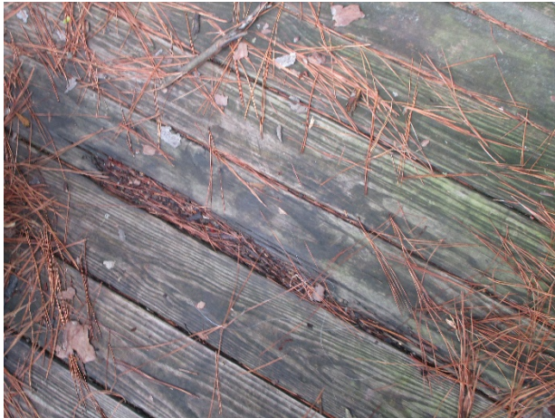
Deck board wood rot
