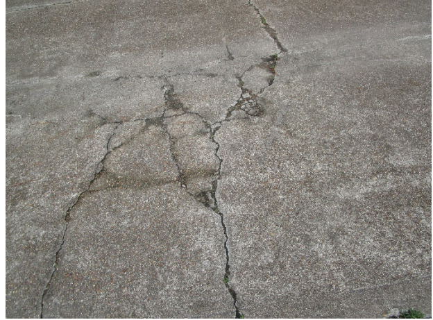
Parking area cracks at the Pinehurst pool
