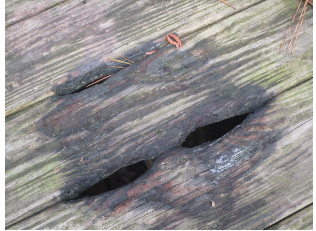
Deck board wood rot
