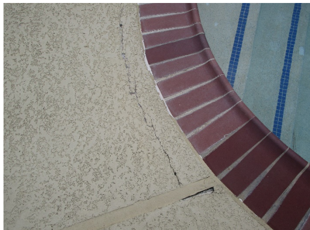
Cracks at the Shores pool deck
