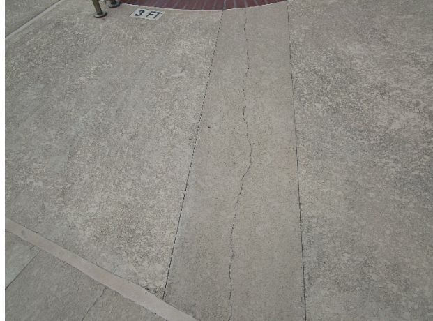
Cracks at the Pinehurst pool deck
