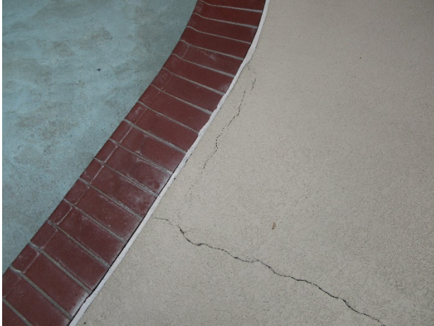
Cracks at the Pinehurst pool deck
