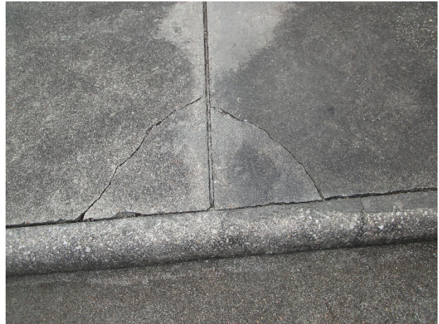
Sidewalk cracks at the Pinehurst pool
