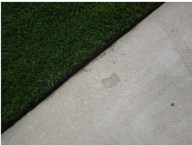
Coating deterioration at the Pinehurst pool deck
