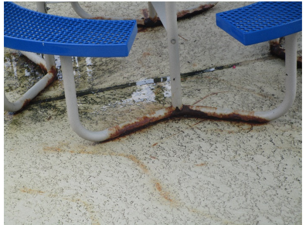
Rust at picnic table
