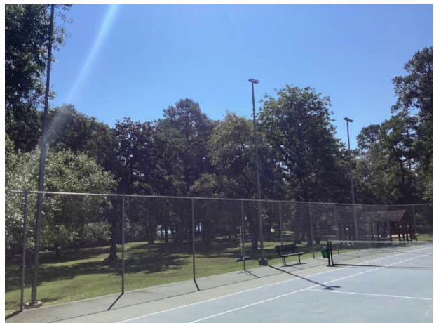
Shores light poles and fixtures
