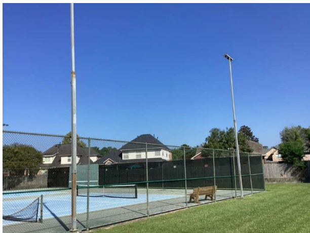
Pinehurst light poles and fixtures
