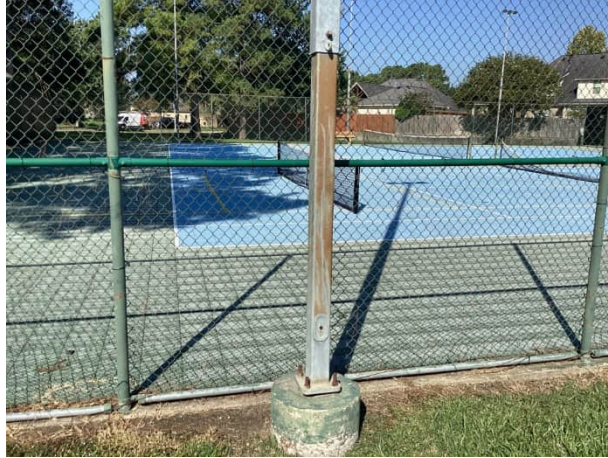
Rust at Pinehurst courts
