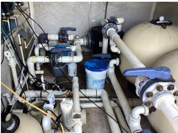
Pool mechanical equipment Pinehurst
