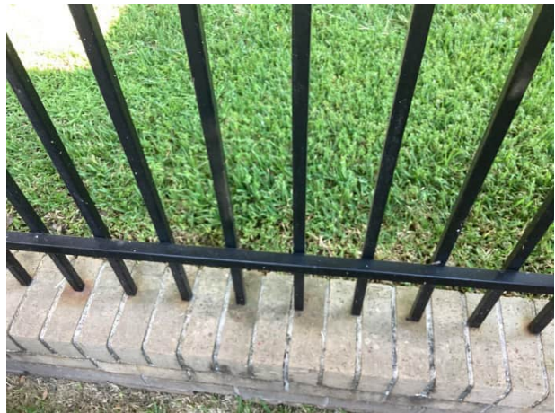
Steel pool fence
