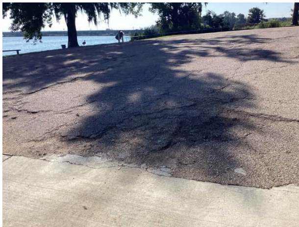
Cracks and deterioration
