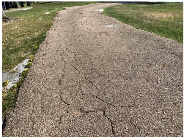
Cracks and settlement
