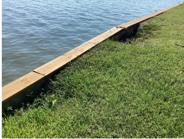
Erosion at bulkhead backside
