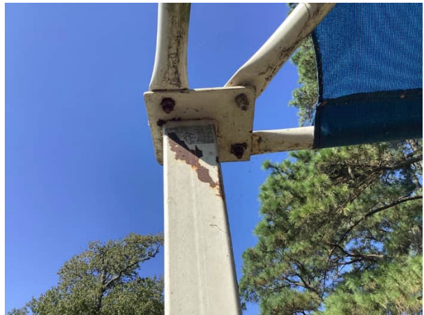
Finish deterioration and fastener rust
