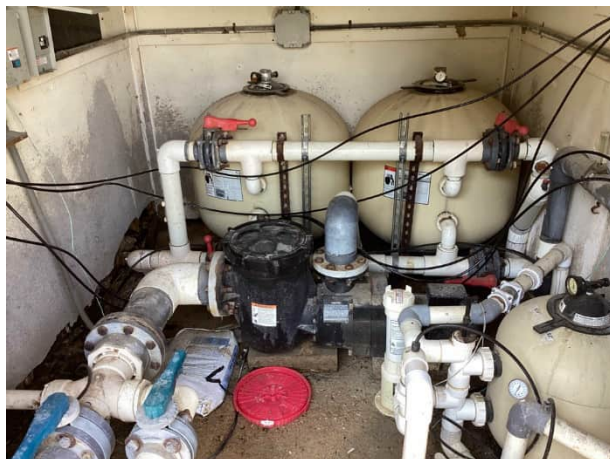
Pool mechanical equipment at Shores
