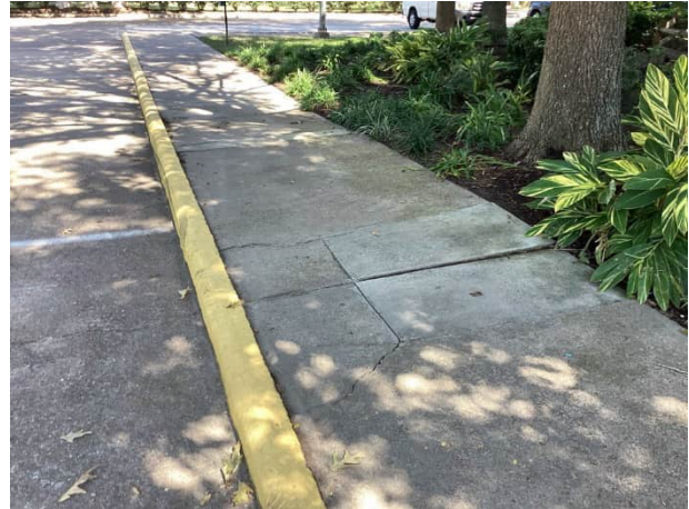
Sidewalk settlement and trip hazards
