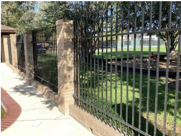
Steel pool fence
